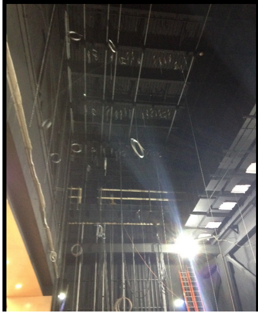
Auditorium Theater Rigging Cables
