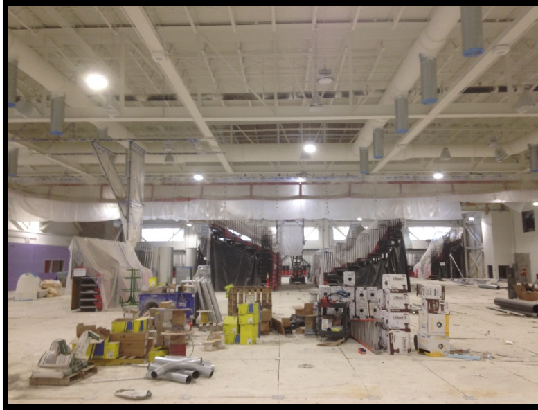
Bldg E Level 2: Light Fixtures
