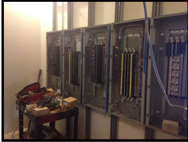
Bldg C Level 1: Electrical Room
