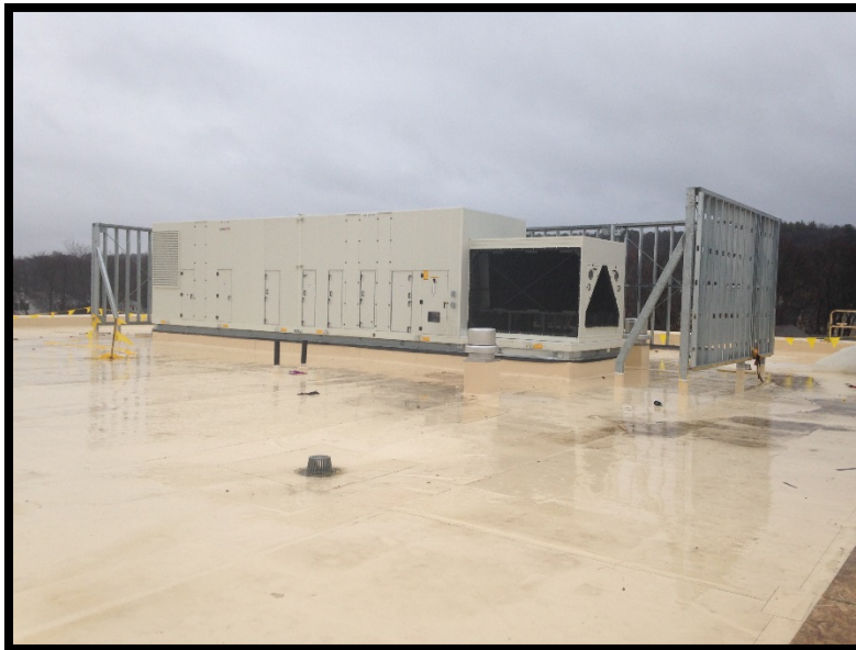
Bldg B Roof: Mechanical Rooftop Unit & Screenwall
