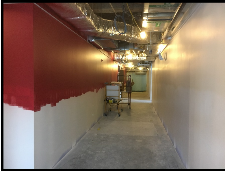
Bldg B Lvl 3: Paint in Corridors
