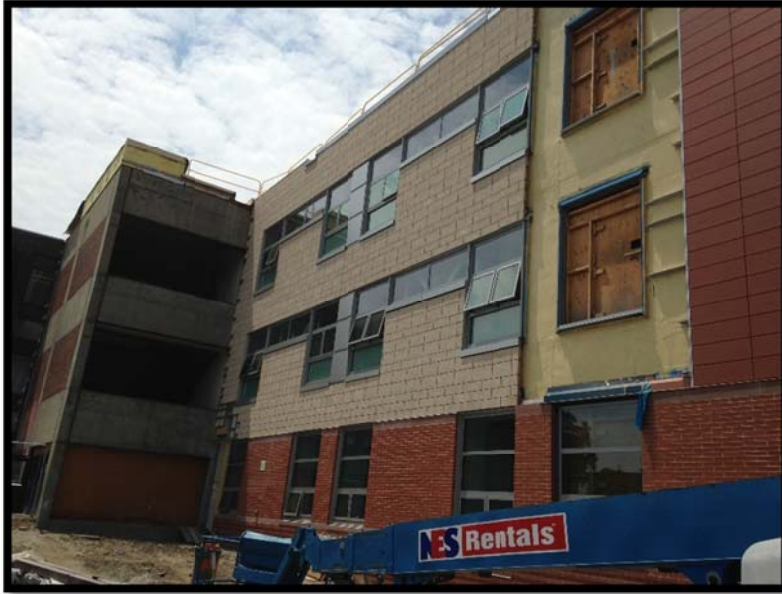
Bldg C East: Demo of Stair C & Install of Windows at Temp Stair
